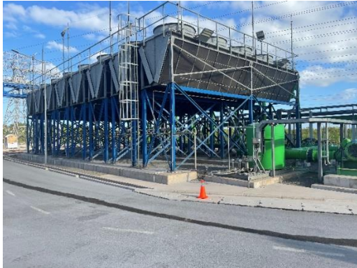
Figura 6: Fin Fan Coolers. [autor]
